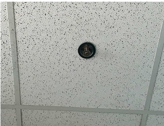
21 - FIRE SUPPRESSION SYSTEM
