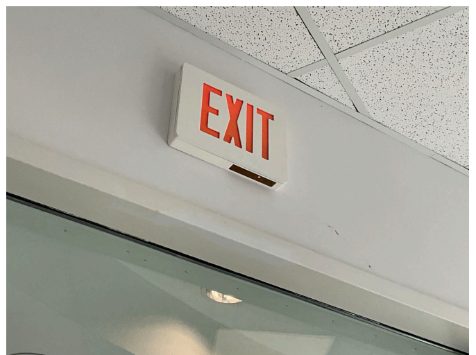
18 - EMERGENCY AND EXIT LIGHTING SYSTEM
