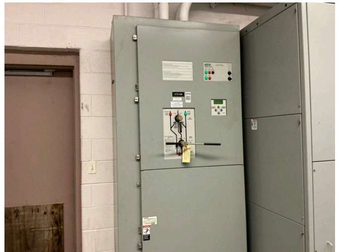
16 - AUTOMATIC TRANSFER SWITCH
