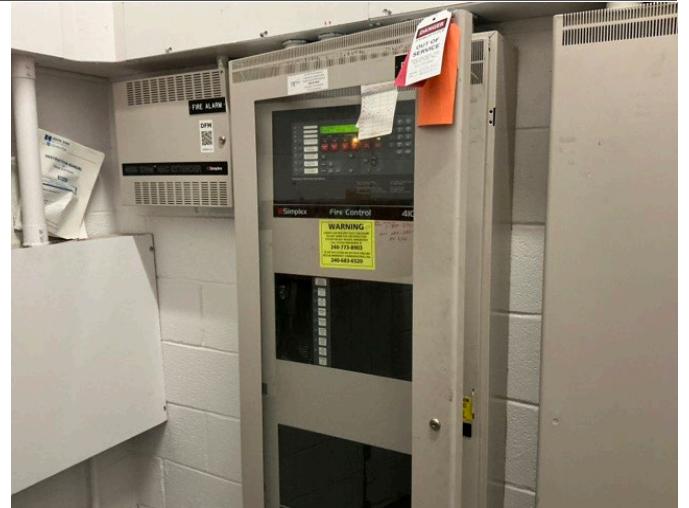
20 - FIRE ALARM PANEL
