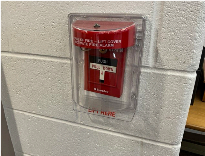
19 - FIRE ALARM SYSTEM
